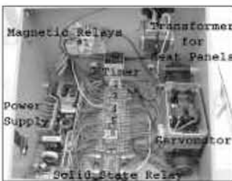
Top: Flipper designer Greg Hoffman wiring the bathroom mirror defrosters.
